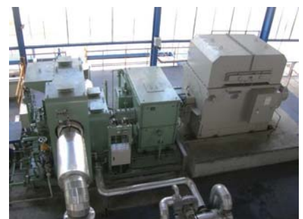
Steam turbine power generator
