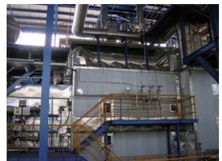
Waste-heat recovery boiler
