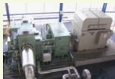
Steam turbine power generator
