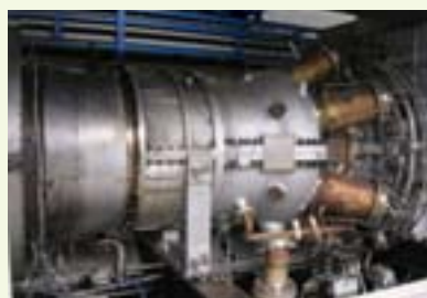
Gas turbine power generator (7,000 kW class)
